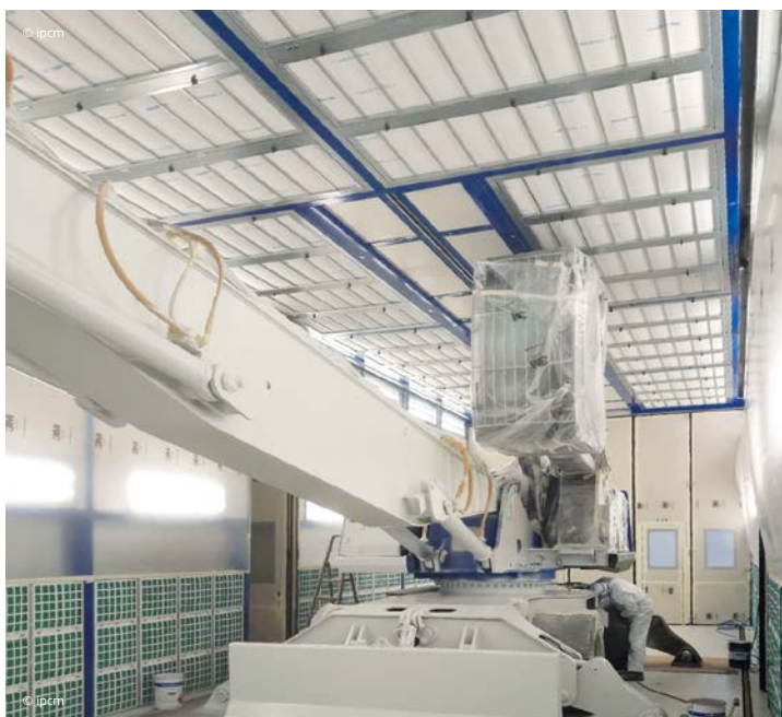
The ceiling of the booth, with a filter deck fed by air-stream burners.
